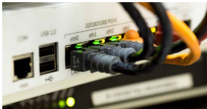
Figure 10.12: Cables connected to a network switch
