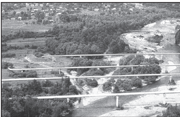
Fig. 8.17: Pipelines transporting natural gas in Ukraine
