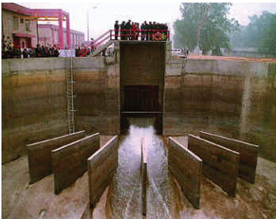
Fig. 18.10 : Water treatment plant
